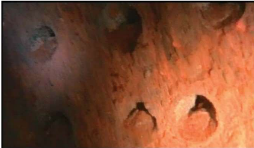
FIGURE 1. Filter porous clogged by salt and metal corrosion products (Photo is taken by Abror Gadaev during the CCTV inspection of the water well filters)
