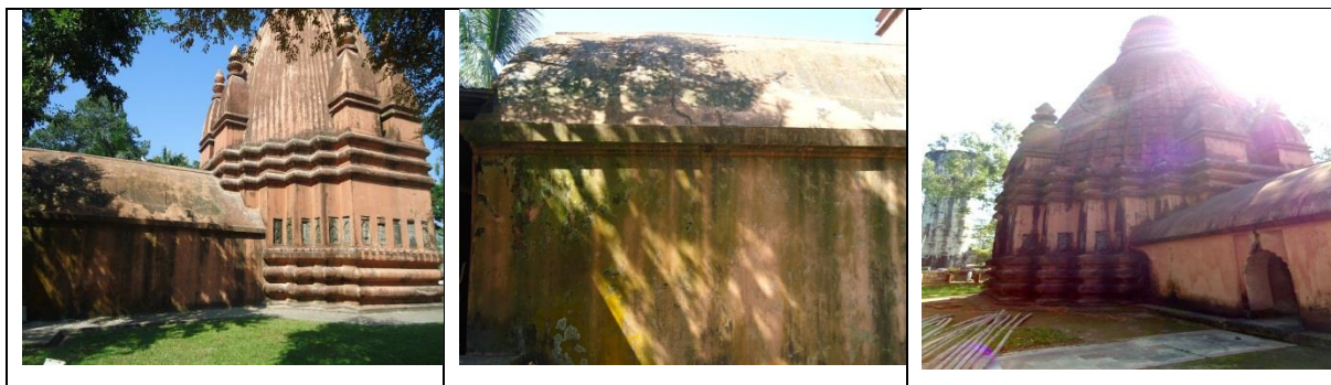
Fig. 1. Lime Plaster North-East Monuments (especially Sibsagar, Assam) shows several conservation problems (Images are self-explanatory conservation problems as discussed in this article).
